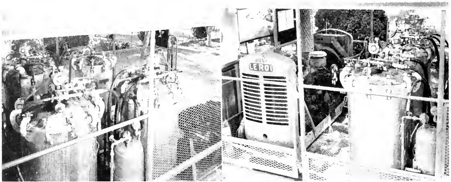
LEFT - Arrangement of point tanks showing air driven mechanical agitators. RIGHT - Close up of compressor and point tanks using air-driven mechanical agitator.
